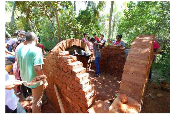
“setting the curve right” - arches have always been a tough task for construction. Students getting a first hand experience of making an arch.
